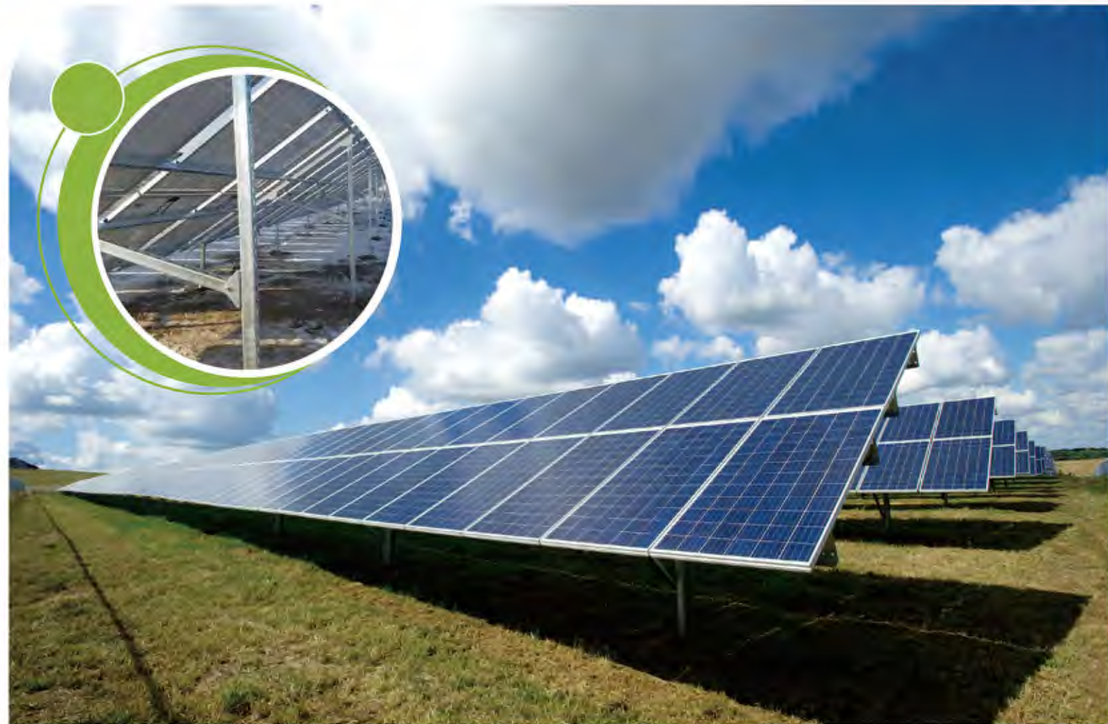
212MW | 新疆库车市 | 固定式支架系统 Fixed Support System 212MW in Kuche City, Xinjiang
