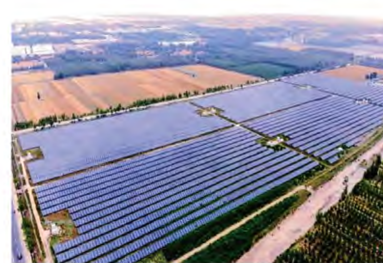
项目地: 山东华电山亭水泉 容量: 150MW 解决方案: 农光互补电站 Project location: Shandong Huadian Shanting Shuiquan Capacity: 150MW Solution: Agricultural Photovoltaic Complementary Power Station
