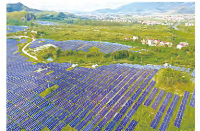
项目地: 江西赣州市于都县 容量: 132MW 解决方案: 固定式支架系统 Project location: Yudu County, Ganzhou, Jiangxi Capacity: 132MW Solution: Fixed bracket system
